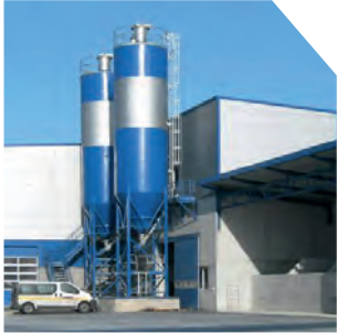
Concrete batching plant
