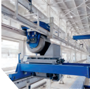
Concrete distribution system
